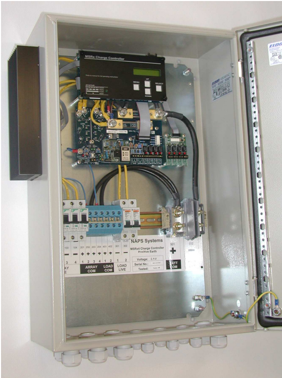
The MSR4 in Painted Steel Enclosure
