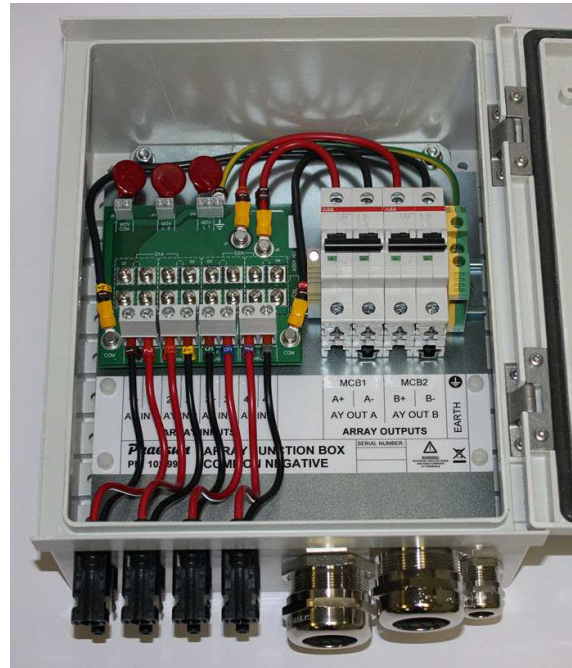
Internal View of Dual Output Unit with MCBs
