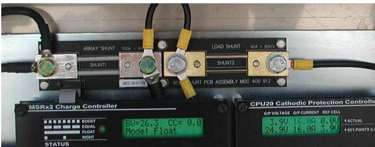
Above photograph shows the shunt assembly fitted inside PN 101103
